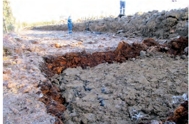
B. Clay has been replaced in the hole where peat had been excavated and placed on top.
