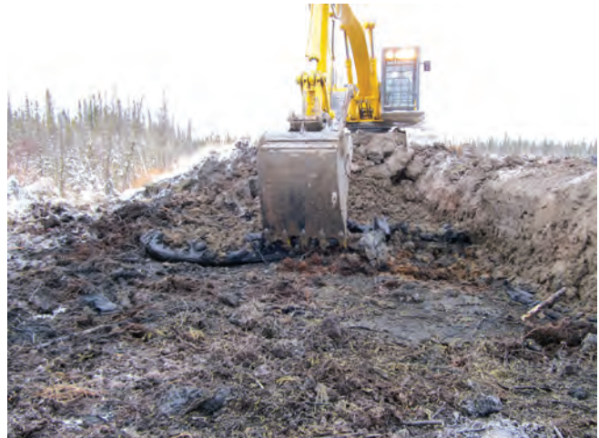
Figure 2. Clay pad material on the right waiting for removal. In the foreground, exposed peat as the geotextile is being peeled back by the hoe. Note the elevation differences between the surface of the clay (right), the exposed peat (middle) and the natural vegetation (left).
